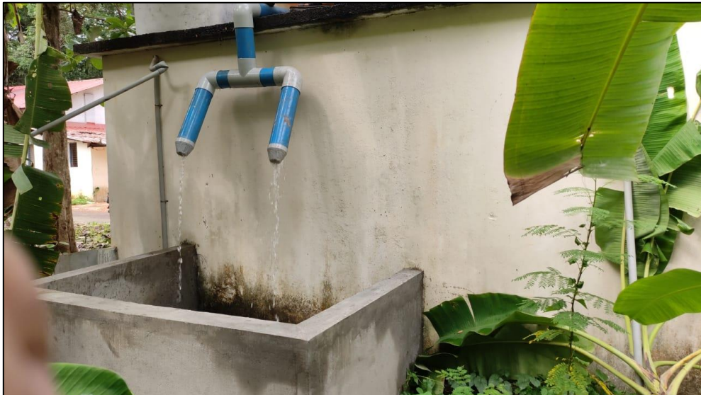
Rain Water Harvesting System at Sree Sankara college, Kalady
