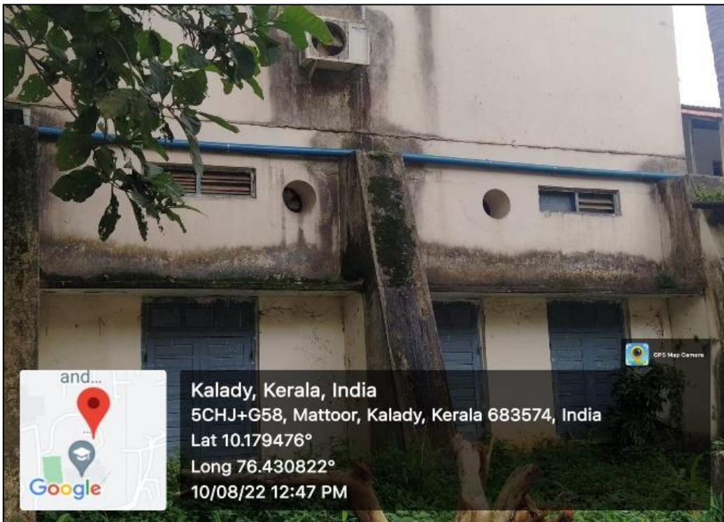
Rain Water Harvesting System at Sree Sankara college, Kalady
